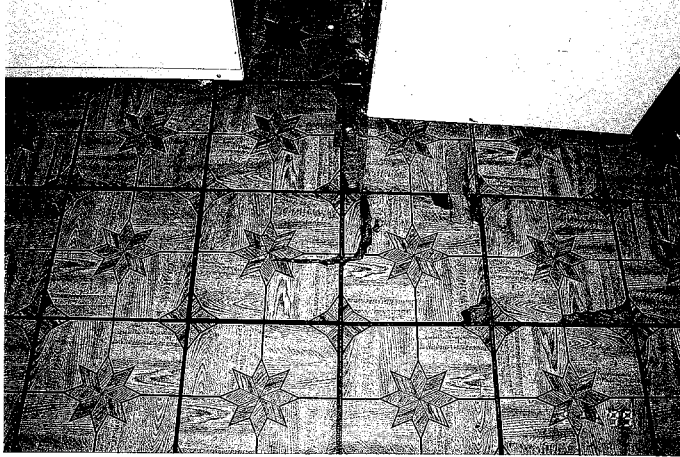
Kitchen floor is damaged.
