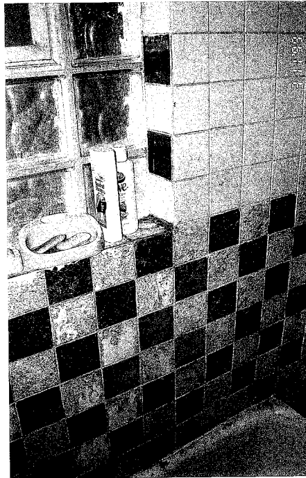
Poor ceramic tile work.
