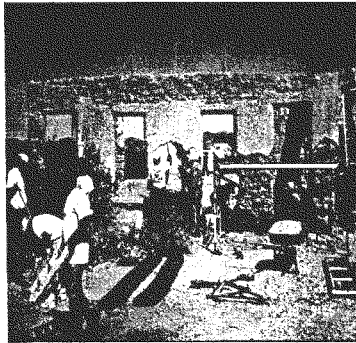
Figure 5 Stabilization work at the Swansea Railroad depot, a project for which BLM Arizona received an Arizona Heritage Preservation Award in 1999
