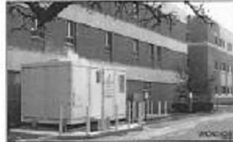
Assured Power South County Hospital Warwick, Rhode Island
