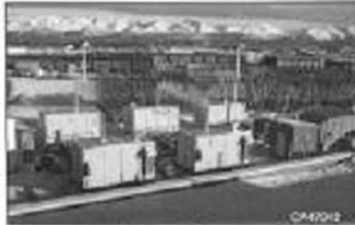
Assured Power U. S. Postal Service Anchorage, Alaska
