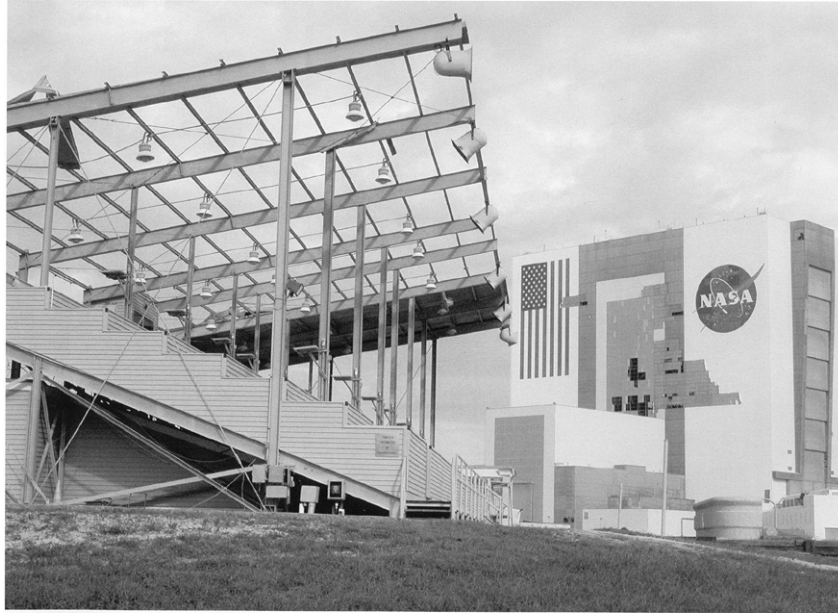
Grandstands—The roof protecting the viewing stands near the Kennedy Space Center press site was blown away during Hurricane Frances. In the background is the Vehicle Assembly Building, which also suffered significant exterior damage during the weekend storm.
