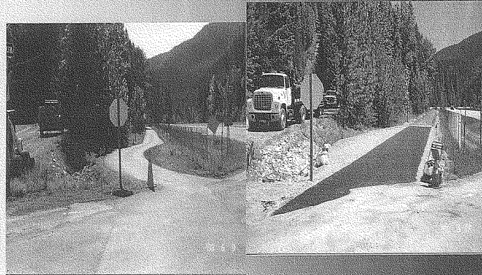
Before and after photos of asphalt repairs to straighten path near Mullan, Idaho.
