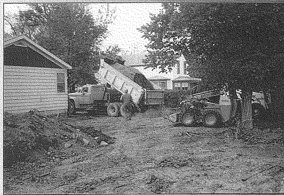
Randall Contracting crews replace contaminated soils at residences near a lead smelter.
