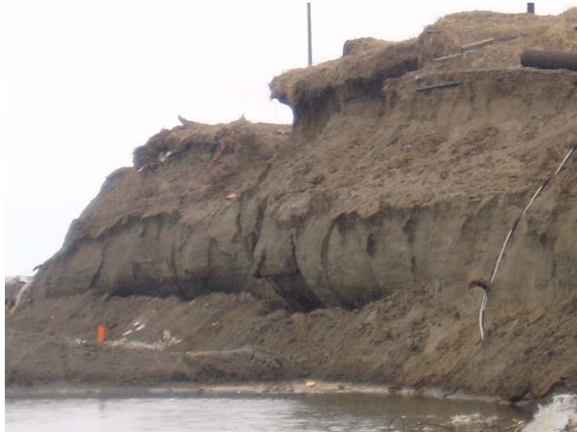
West end permafrost exposed and melting
