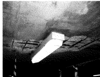
Spalling Garage Roof
