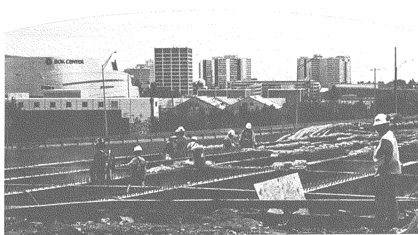
Oklahoma DOT is using $65 million of its Recovery Act funds to reconstruct I-244 in Tulsa.
