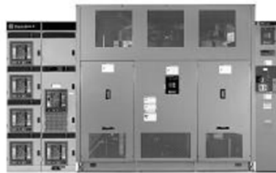
Figure 3—Distribution Transformer with Built-in Webserver.
