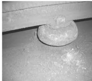
Extremely dirty insulator
