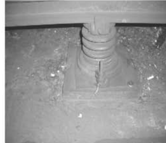
Insulator close to failure
