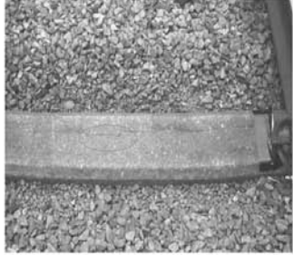
Cracked concrete tie due to rebar corrosion from leakage current
