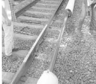
Failed Insulator plasma ball distorted rails
