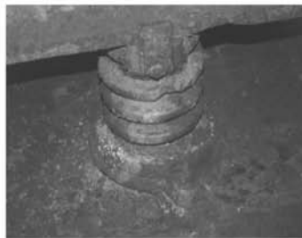
Dirty insulator close to failure
