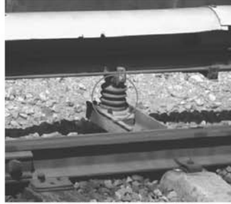
Typical Dirty Insulator
