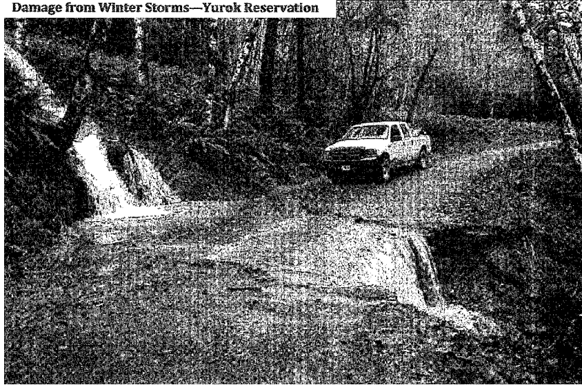
Damage from Winter Storms—Yurok Reservation
