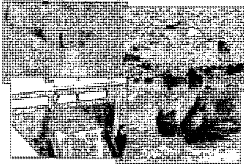
Figure 3: Examples of Deferred Maintenance on BIA's Irrigation Projects (c. 2005)
