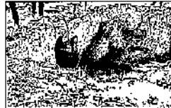
Crumbling Concrete Structure
