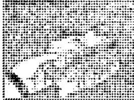
Concrete that Fell from Flume
