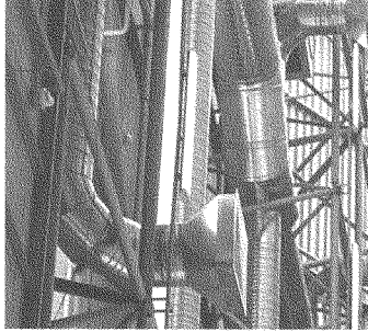
Heating, ventilation, and air conditioning (HVAC) applications
