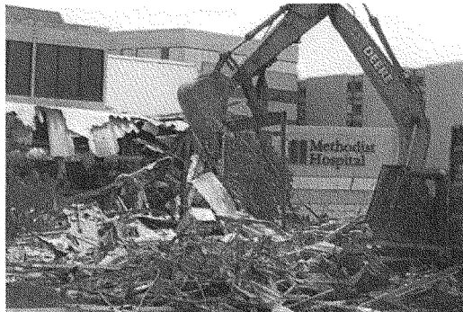
Demolition of a building on the Methodist Hospital campus was photographed July 5, July 5 2011 John McCusker, Times-Picayune archive
