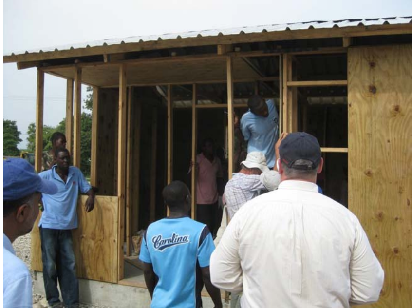
Fig. 6: “T-shelters,” semi-permanent transitional shelters, are being constructed at many relocation sites, including at the Tabarre Issa Emergency Relocation Camp. While durable, the T-shelters have been more expensive than budgeted, and their construction has been delayed due to supplies being held up by Haitian Customs officials. It has been estimated that 125,000 T-shelters have been donated (which could house up to 600,000 people), but the land upon which to build and place them has yet to be identified by the Government of Haiti. June 8, 2010
