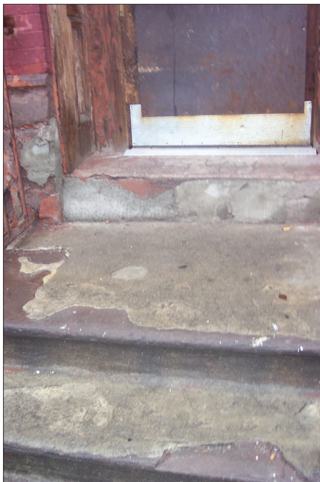
Figure 22: Property 4—$3,978 in Stoop “Repairs”
