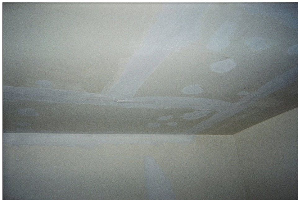
Figure 18: Property 3--“New” Kitchen Ceiling
