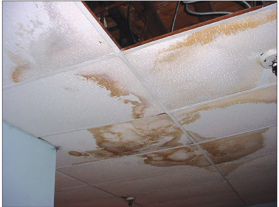
Figure 11: Property 1—“New” Ceiling
