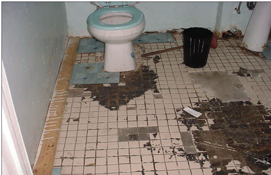
Figure 12: Property 1–“New” Bathroom Floor
