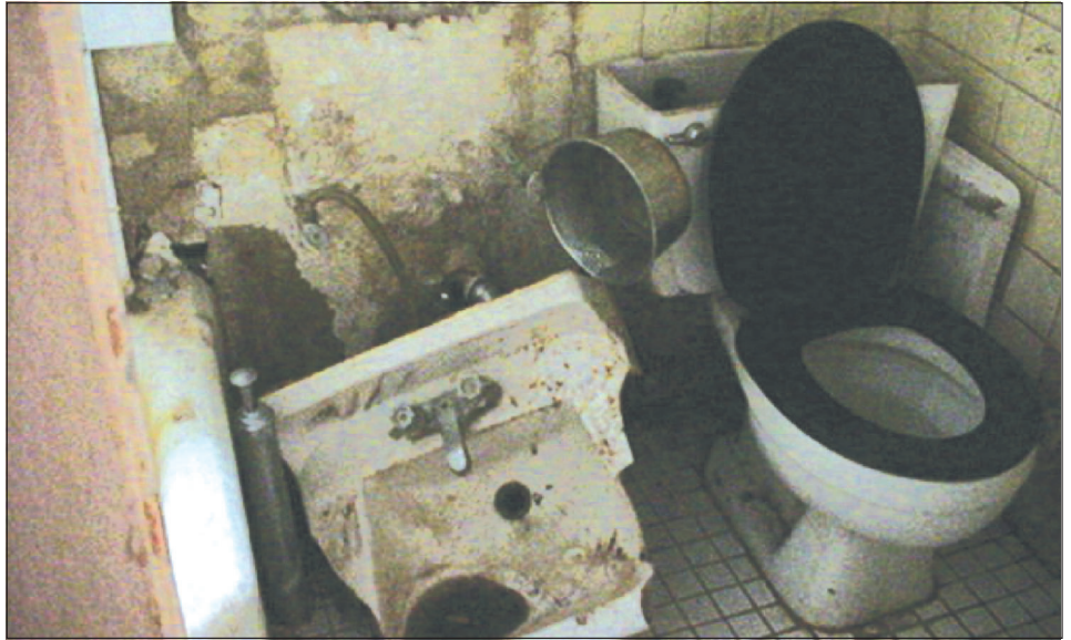
Figure 16: Property 2—More Bathroom “Repairs”
