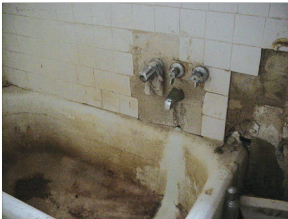
Figure 15: Property 2–Bathroom “Repairs”
