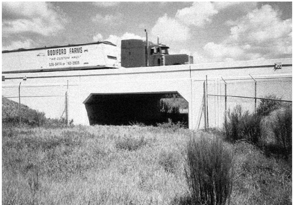
Figure 3: Example of an Underpass Created to Allow Bears to Cross Highway Right-of-way without Danger of Collisions with Vehicles
