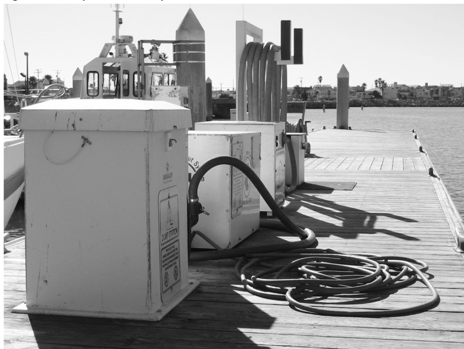
Figure 2: Pumpout and Dump Station in Channel Islands Harbor, California
