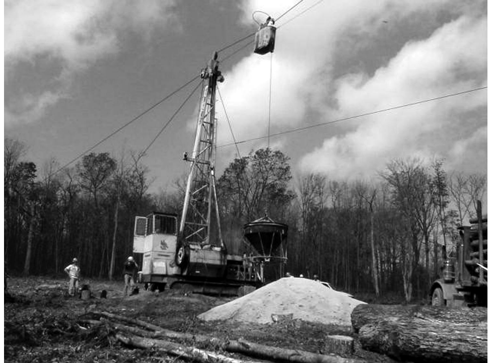
Figure 4: Limestone to Be Added to a Creek to Reduce Acidity at the Burns Creek Pilot Project, George Washington-Jefferson National Forest
