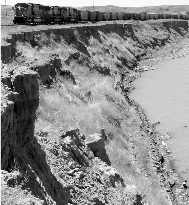
Figure 18: Caving Streambed along a Railway Posed a Safety Hazard
