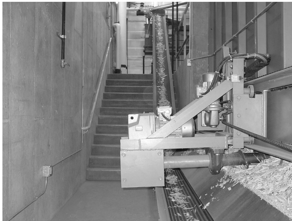
Figure 5: Automated Wood Chip Conveyor, Darby School District Project, Darby, Montana
