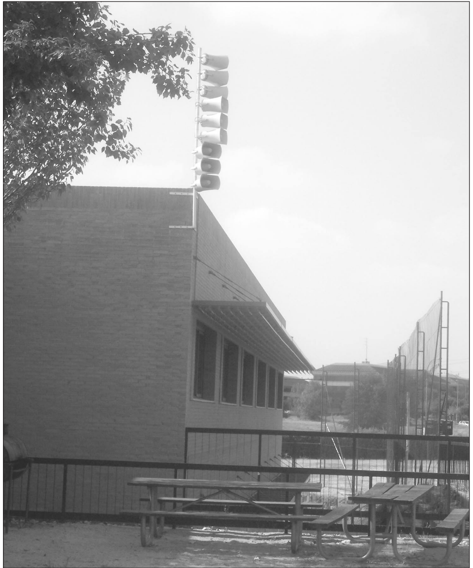
Figure 5: New Public Address System Funded by the Soft Targets Program
