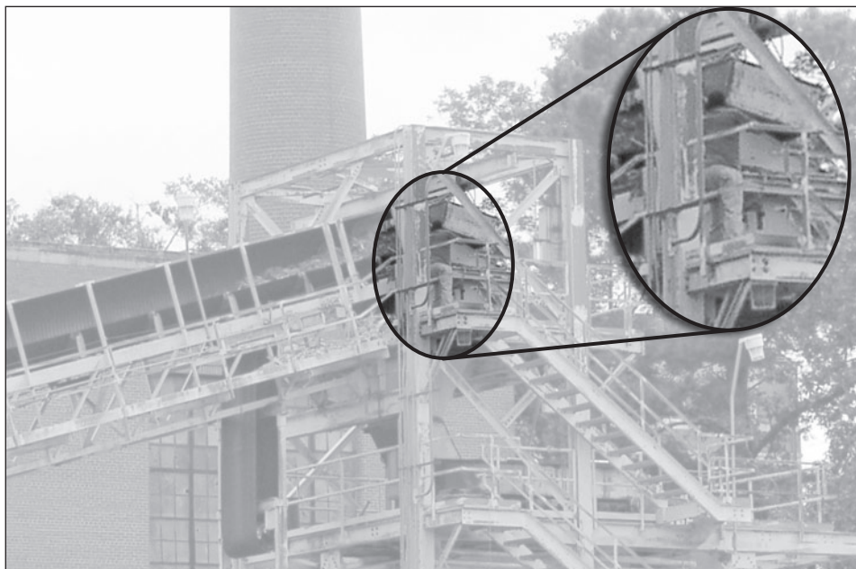
Figure 4: Maintenance Crew Member Clearing Wood Blockage in Conveyor Equipment
