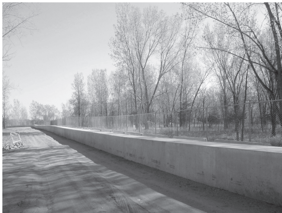
Figure 3: Example of a Vehicle Barrier System
