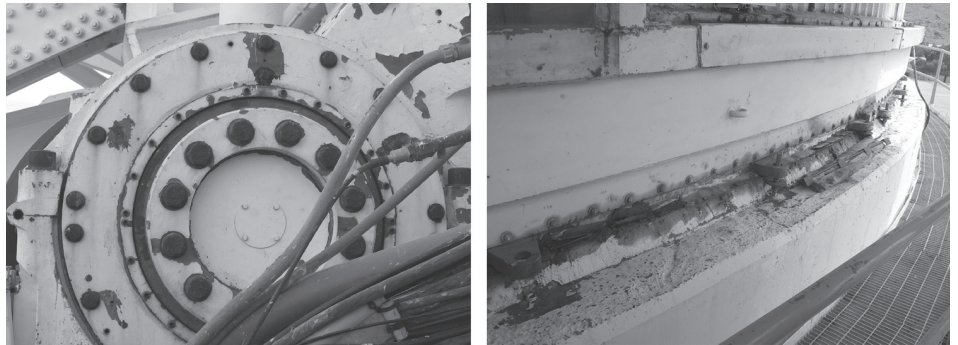
Figure 2: External corrosion on 70-meter antenna
