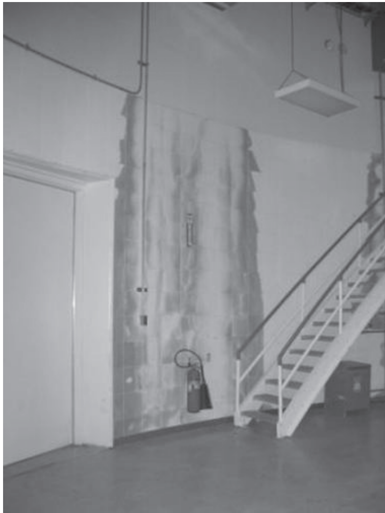
Figure 4: Water Intrusion to Internal Antenna Structure at Goldstone Facility
