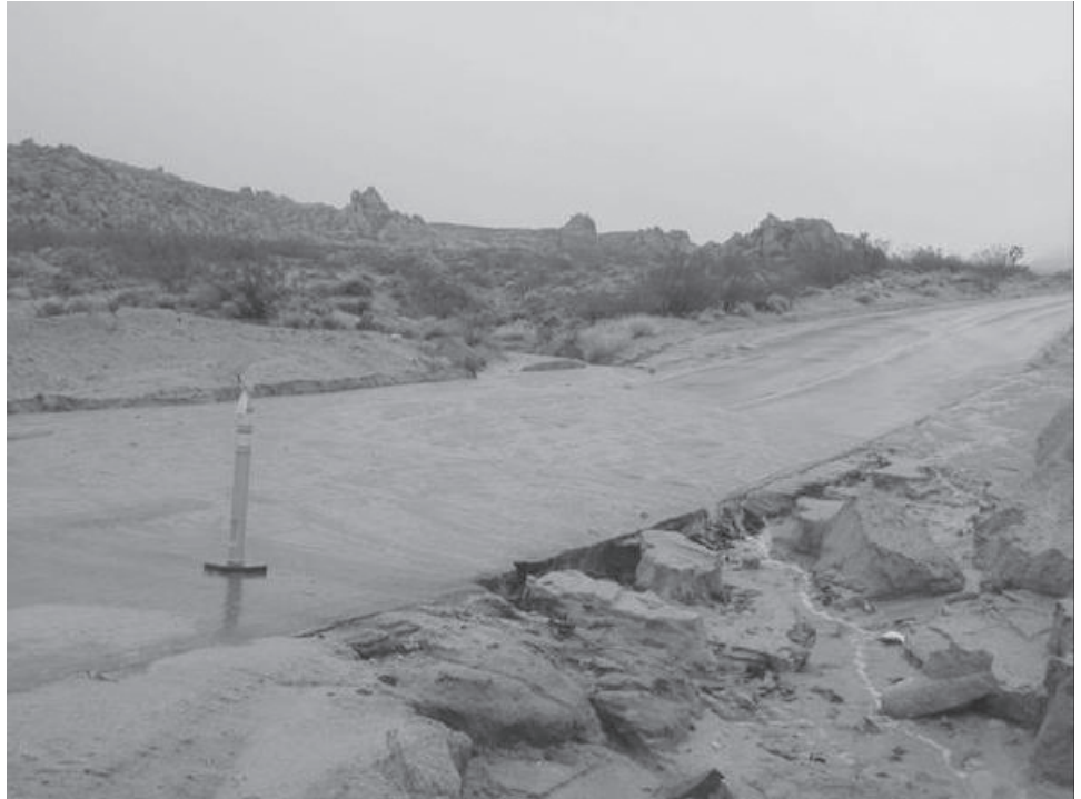
Figure 3: Road Damage to Asphalt Roadway at Goldstone Facility
