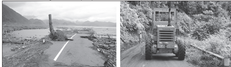
Tsunami-Damaged Road (left) and USAID-Funded Maintenance Work in Indonesia
