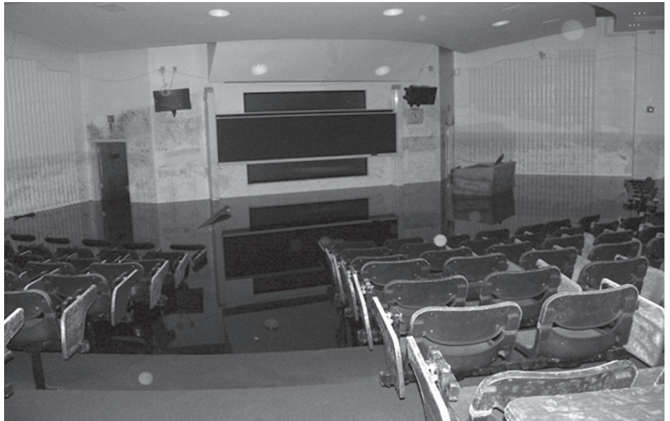
Figure 2: Xavier University Science Building Auditorium Before and After Restoration from Flood Damage
