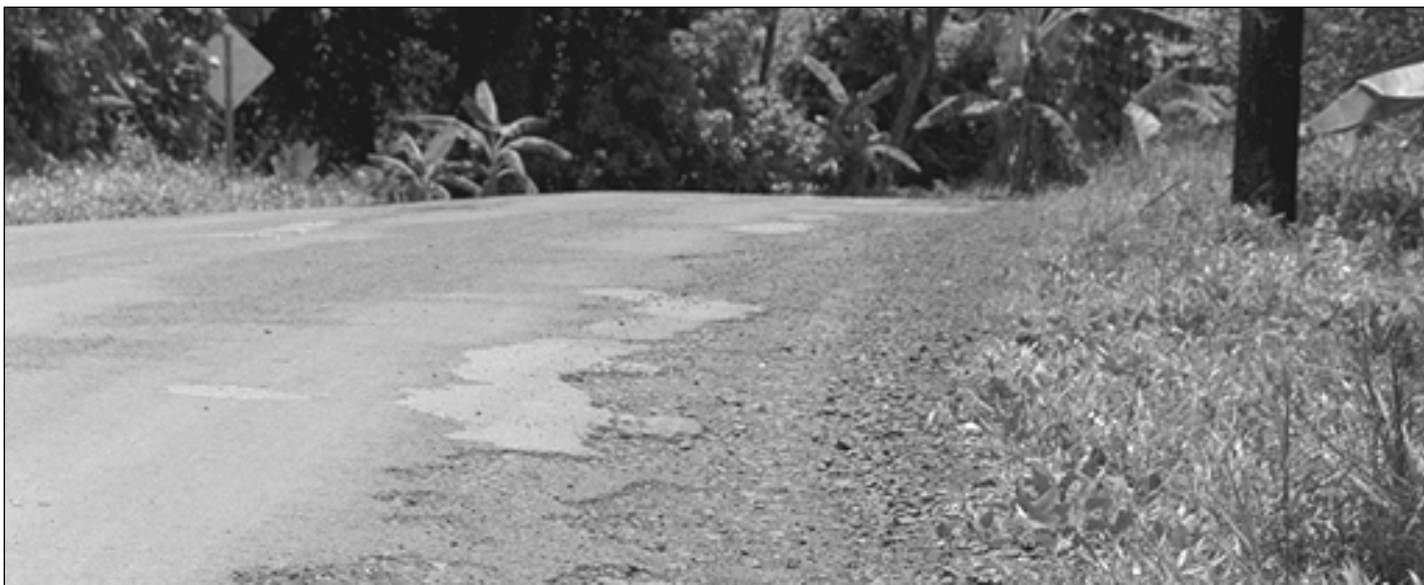
Eroded Asphalt Shoulder
