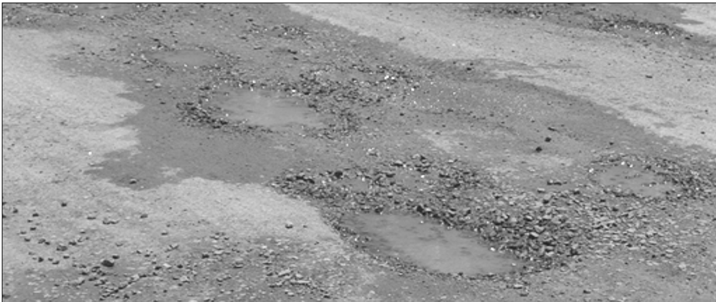
Potholes in Road Base
