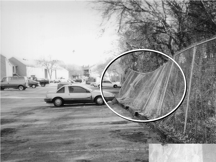
Figure 2: Physical Conditions That REAC Quality Assurance Reviewers Found Contract Inspectors Did Not Record at Properties GAO Visited
