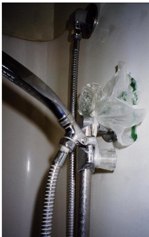
Plastic bag holding broken shower facility
