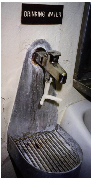
Corroded drinking water facility and damaged wall
