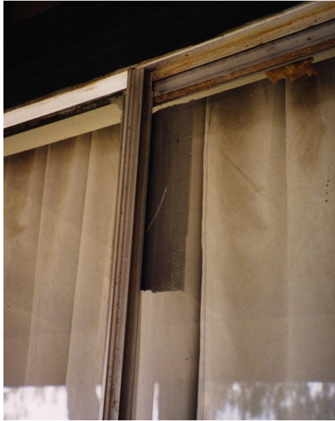
Duct tape on broken window
