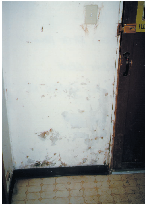
Mildew on shower wall
