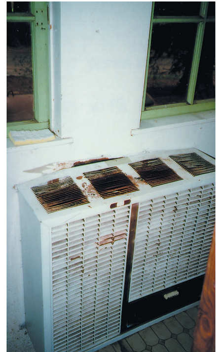
Rusty heater fixture
