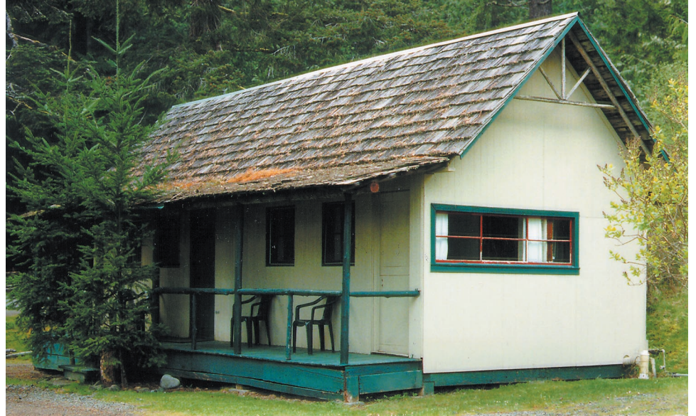
Figure 6: Needed Exterior Repairs at Log Cabin Resort
