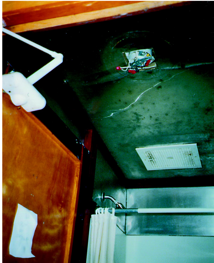
Figure 10: Exposed Wiring in Public Bathroom and Shower Facilities
