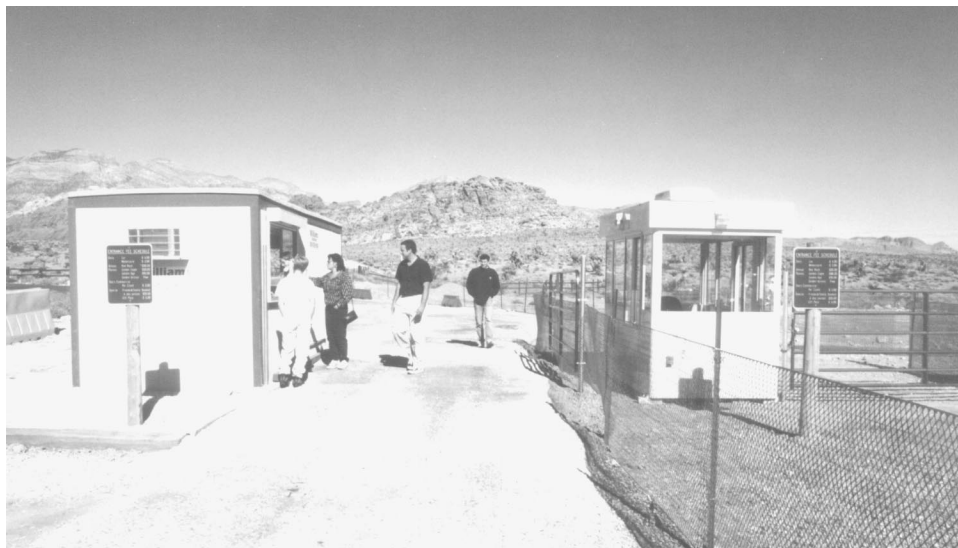
Figure 2.3: New Entrance Station Under Construction at Red Rock Canyon—a BLM Demonstration Site in Nevada
