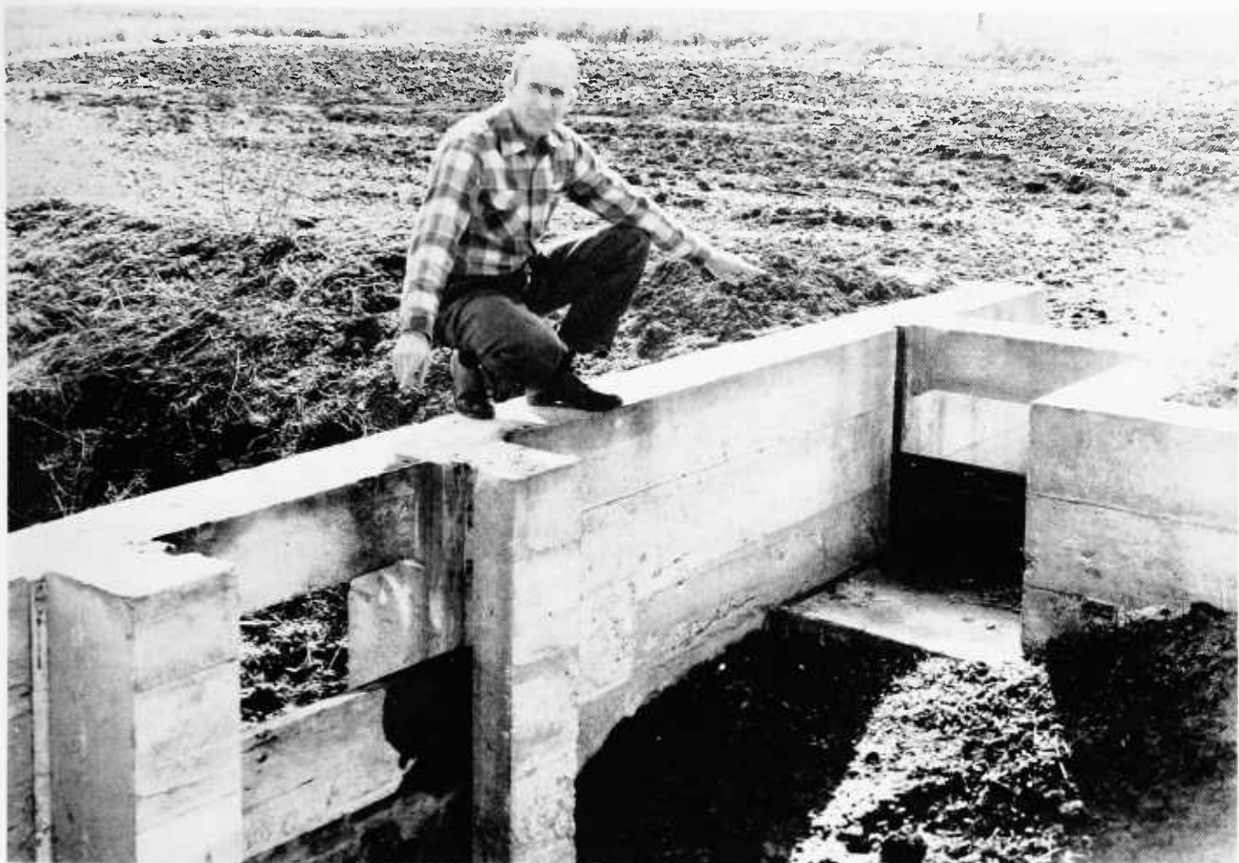
FIGURE 34.—Headgate that controls flow of water from canal into ricefield.
