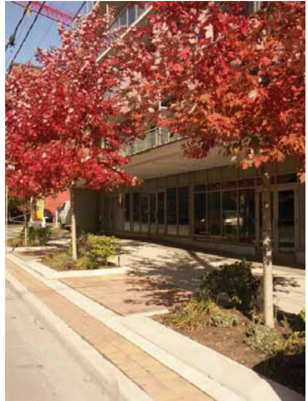
Continuous soil trench construction to provide Toronto street trees with increased soil volume. Photo by Urban Forestry, City of Toronto, used with permission.
