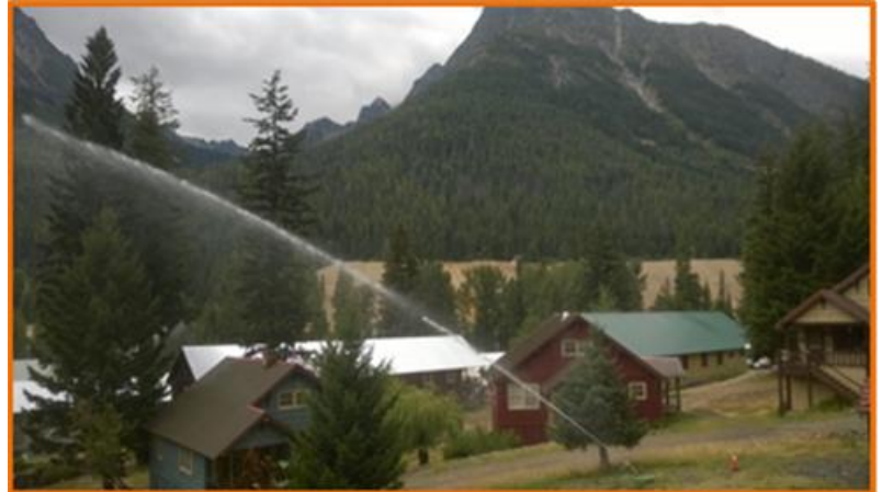
Sprinkler system established for structure protection at Holden Village.
