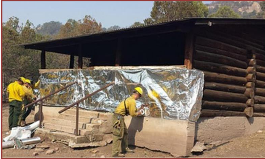
Firefighters wrap the historic Gotchen Cabin, built in 1909 on the Gifford Pinchot National Forest, to protect this structure from the approaching Cougar Creek Fire. This protective material is special aluminized structure wrap. Photo courtesy U.S. Forest Service.
