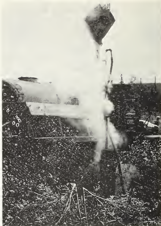
FIGURE 1 – Extraction of steel pile in permafrost at Fairbanks, Alaska. Soil was thawed by advancing a steam jet adjacent to and down to the depth of the pile until the pile heaved up.
