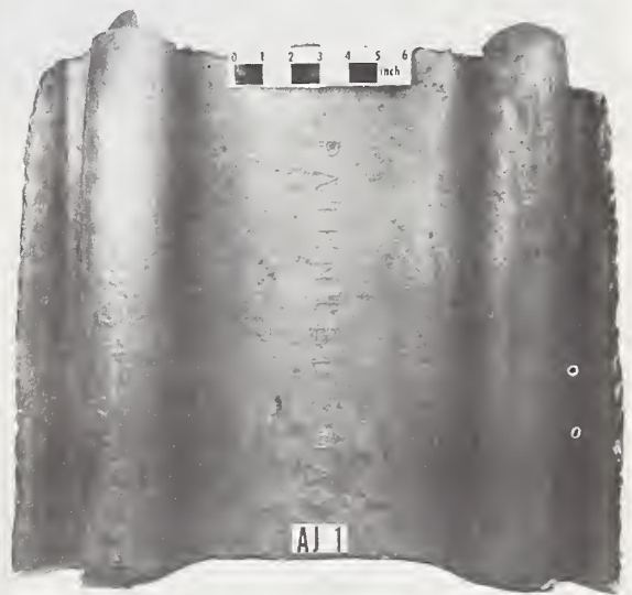
FIGURE 3 – Section of steel sheet-pile pulled from an engineer’s slip on the Niagara River at Buffalo, N. Y., after exposure for 36 years. The section was exposed about 8 ft below the ground line in the water table zone.
