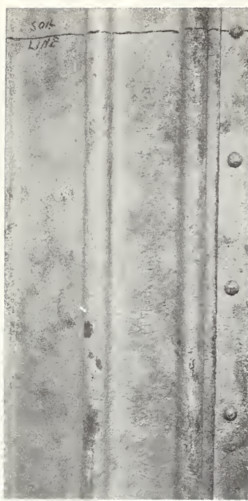
FIGURE 4. A 3-ft section of steel sheet piling exposed below the soil line in a cofferdam structure in the Lumber River near Boardman, North Carolina.
