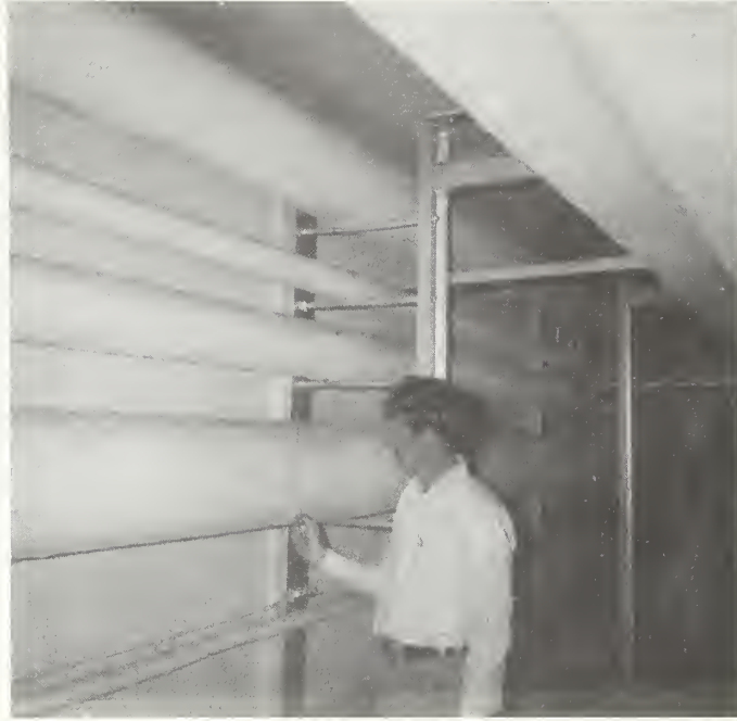
Figure 13 Interior of the walk-through utilidor at Ft. Wainwright, Alaska (Photo by R. Redfield, USACREEL).
