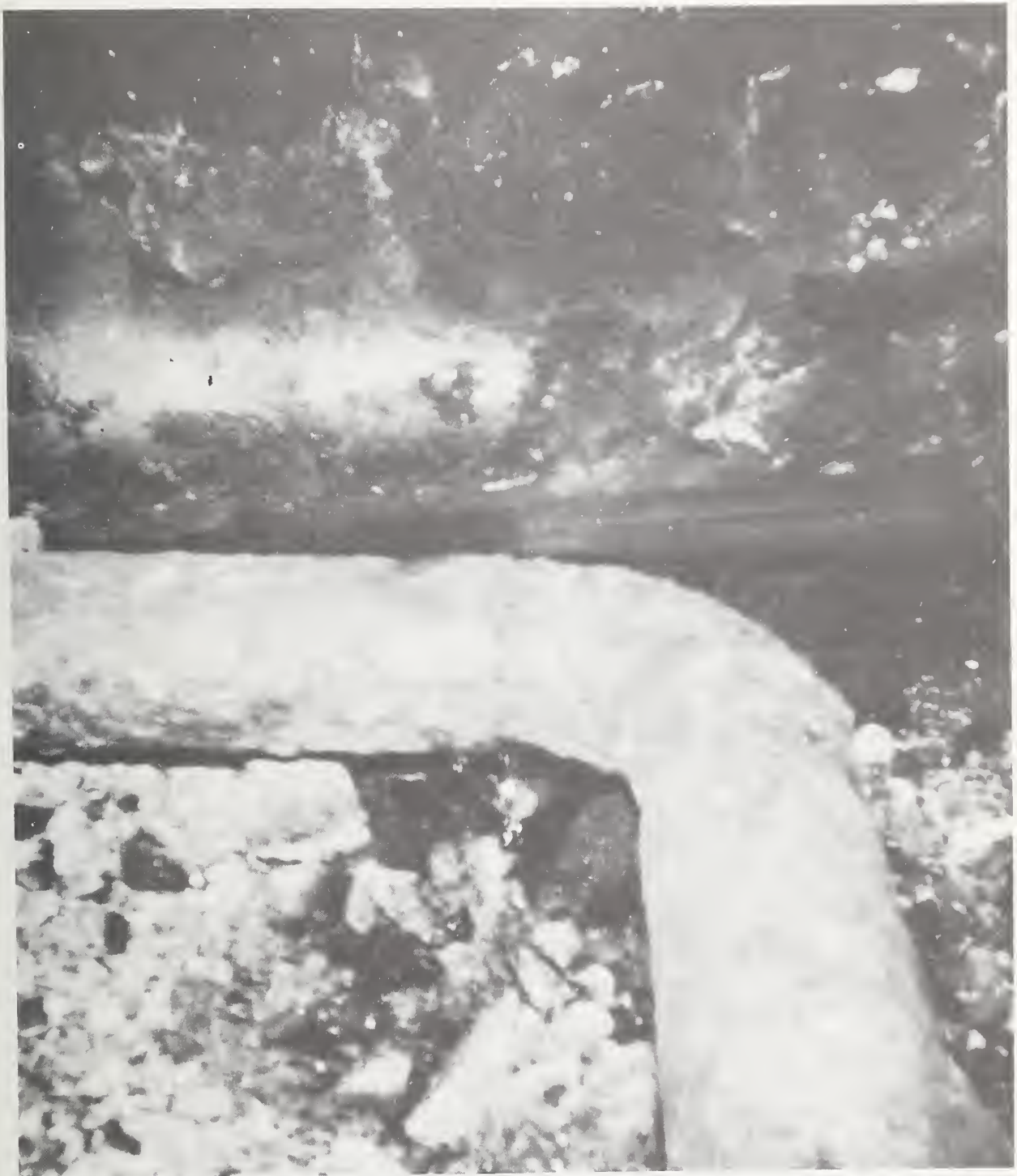
Figure 5 Corroded Condensate Piping Installed in Hydrocarbon Backfill.
