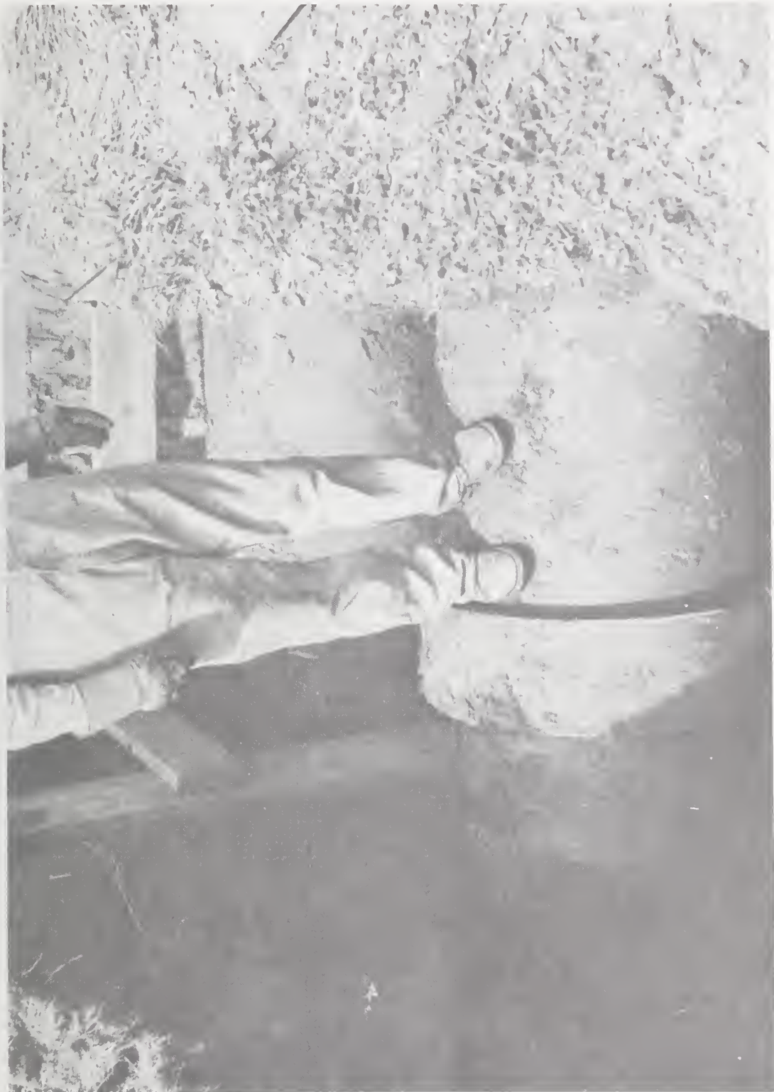
Fig. 8 CEMENT ASBESTOS CHILLED WATER PIPES BETWEEN THE PENTAGON AND FOB #2 EXCAVATED FOR THE HEAT FLOWMETER INSTALLATION
