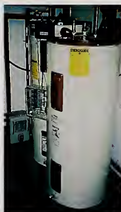
Top: Solar collection array Bottom: Solar powered domestic water heater
