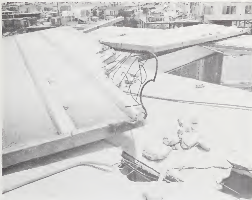
Fig. 14. Overturned ceiling panels - CGI cladding and roof framing completely removed.
