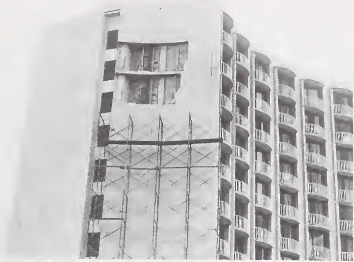
Fig. 29. Travelodge - Darwin City (similar damage at opposite end)
