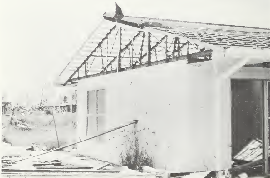
Fig. 16. Prefabricated house with asbestos cement-polyurethane sandwich panels and steel wall and roof frames
