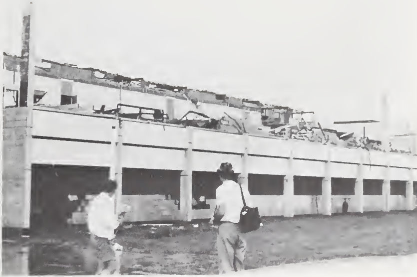
Fig. 21. Failure of second story (view immediately to right of Fig. 20)
