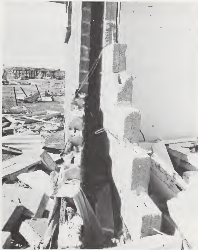
Fig. 10. Failure of brick and concrete block cavity wall
