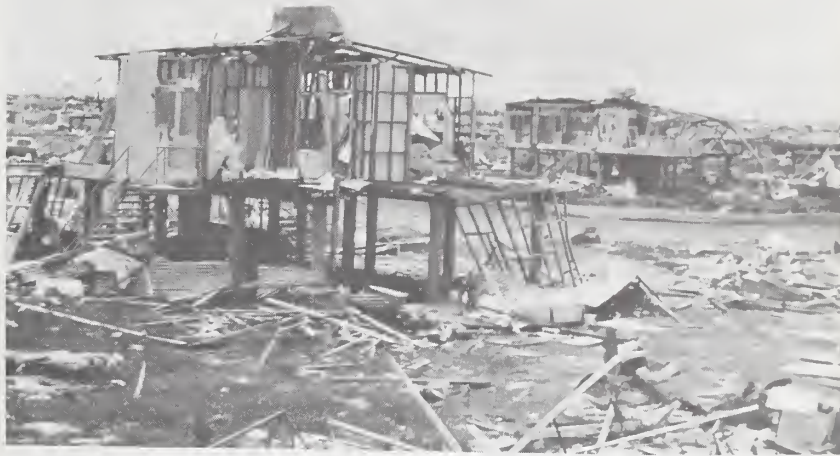
Fig. 9. Failure of endwall
