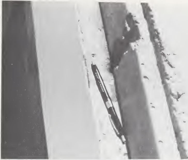
Fig. 13. Ceiling panel anchorage - bolt and adjacent panel missing
