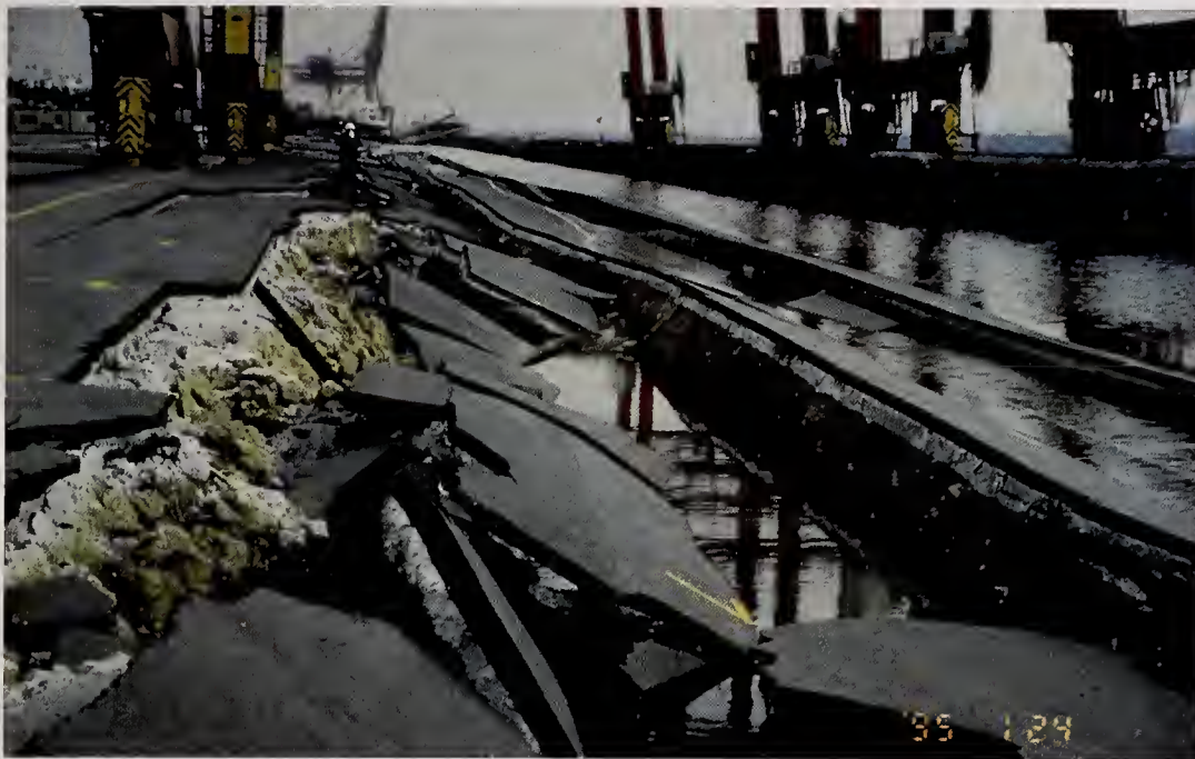
Damaged port facilities in Kobe, Japan caused by liquefaction
