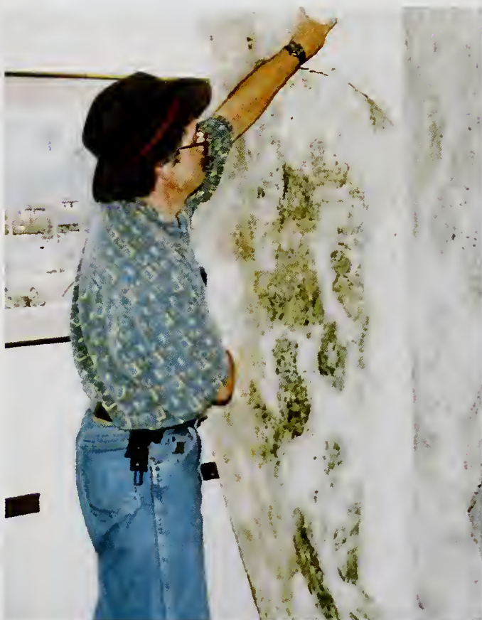
Mold and mildew as a result of poor moisture control
