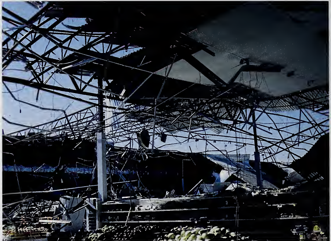
Damaged Interior of the Albertsons store in Williamson County, Central Texas after being hit by the F-3 Cedar Park Tornado
