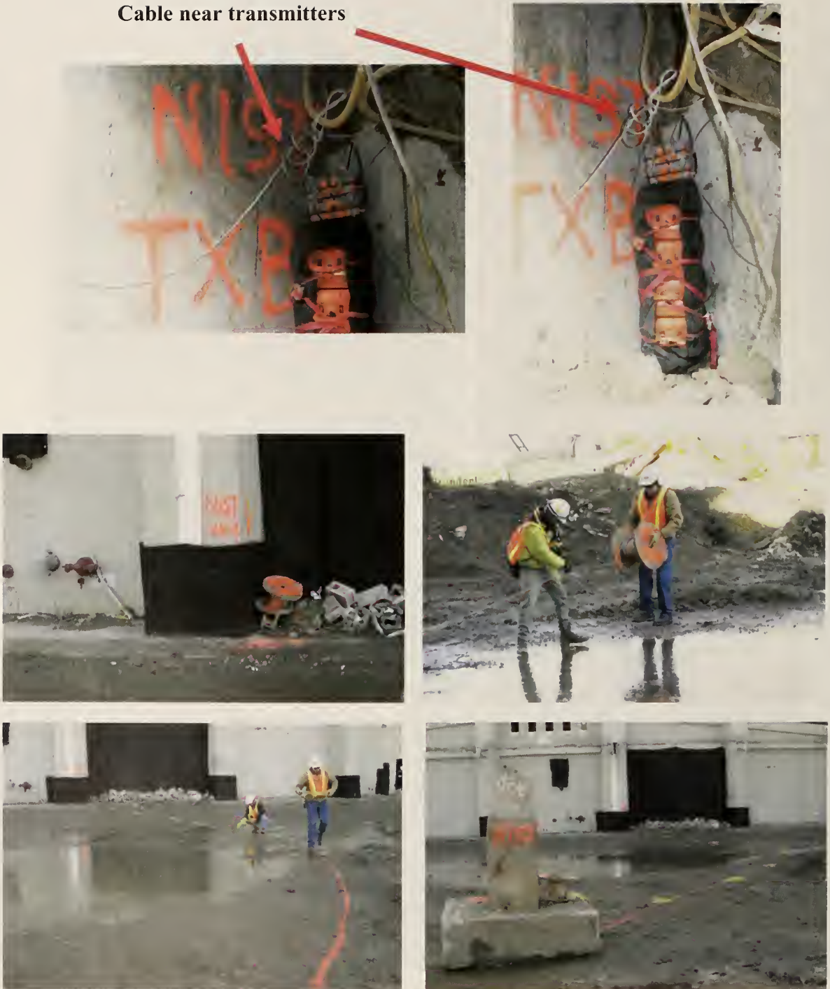
Figure 22. Cable on north side of stadium. This cable was run from the transmitter site on the playing field (TX B).
