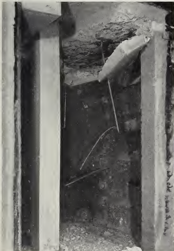
FIGURE 12. Column protected with milky quartz aggregate concrete after 3-hr 10-min fire exposure—Test 3.
