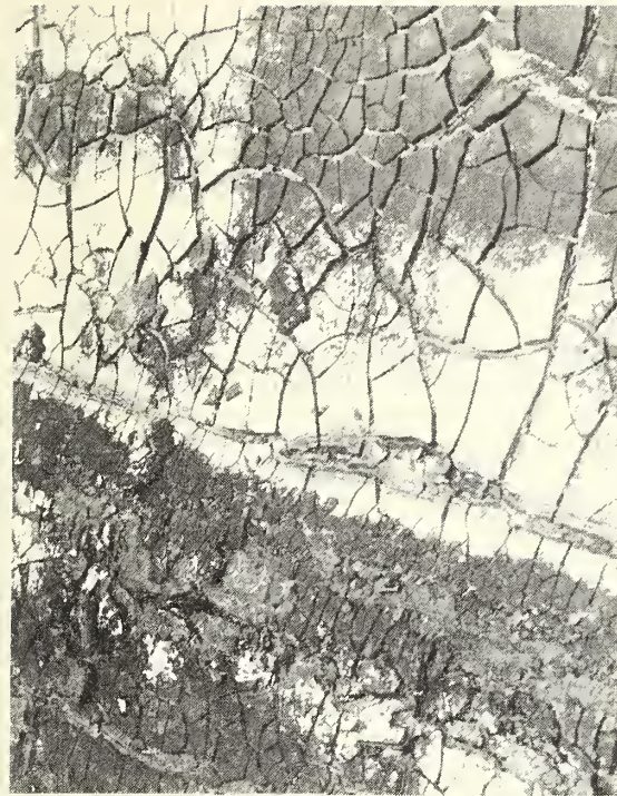
FIGURE 10. CONDITION OF WEATHERED BITUMINOUS ROOFING BEFORE REMOVAL.
