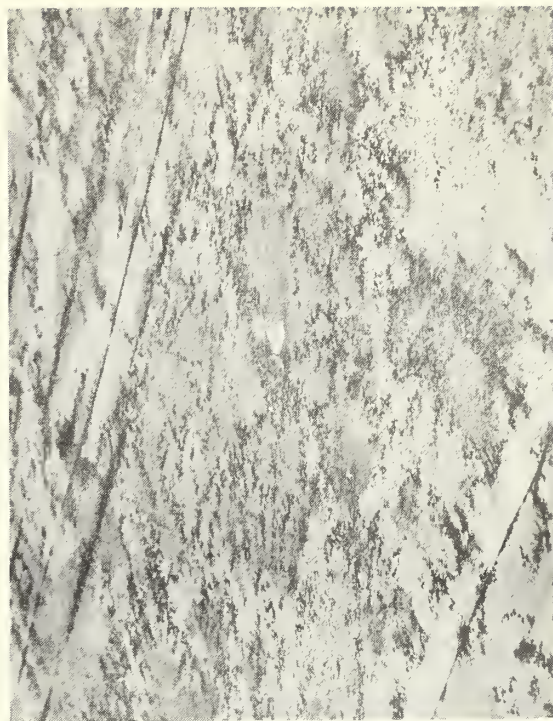
FIGURE 8. CONDITION OF REINFORCED MEMBRANE SYSTEM SHOWING MILDWE GROWTH. AGE 75 MONTHS.
