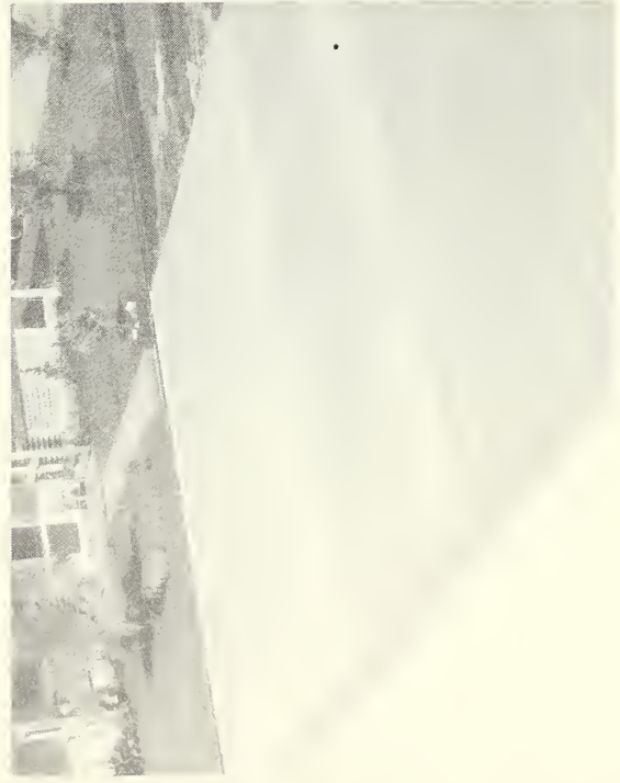
FIGURE 15. DISCOLORATION OF BUTYL SHEET ROOFING ATTRIBUTED TO USE OF INCOMPATIBLE MATERIALS.
