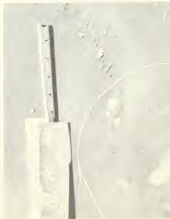
FIGURE 7. BLISTERING AND SALT DEPOSITS ON EMULSION COATING. AGE 45 MONTHS.
