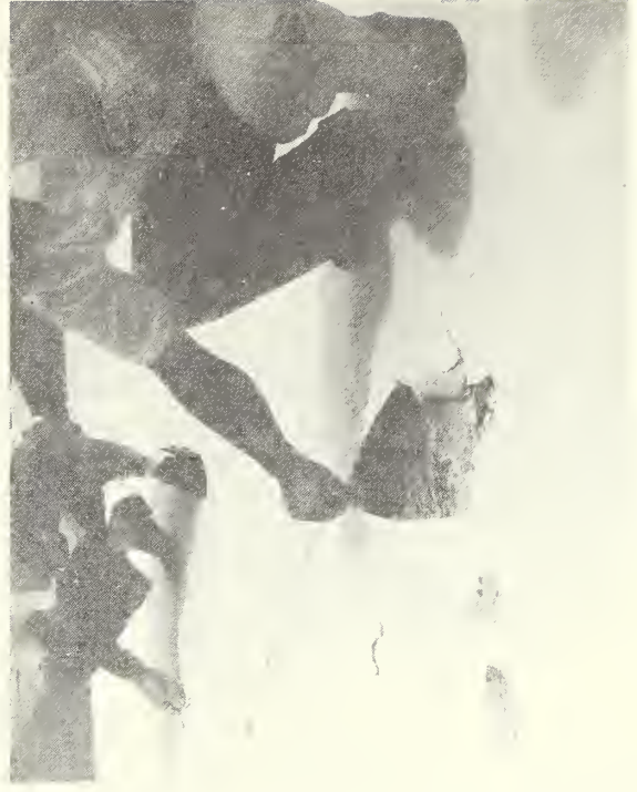
FIGURE 16. DEFECTS IN FLUID-APPLIED SYSTEM ATTRIBUTED TO POOR PREPARATION OF CONCRETE DECK
