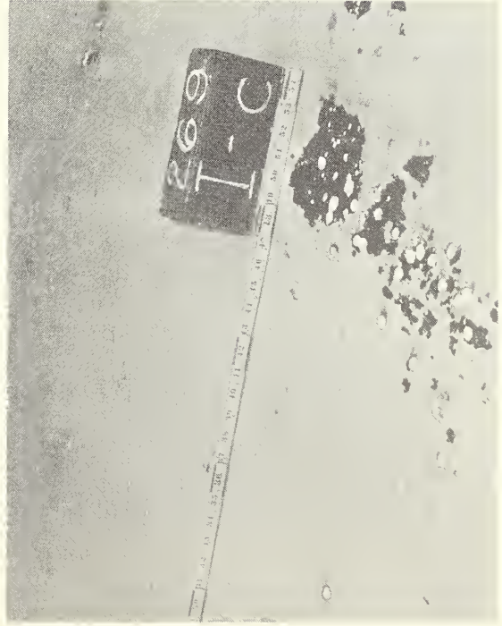
FIGURE 3. GENERAL DETERIORATION OF AN ALUMINUM COATING. AGE 38 MONTHS.
