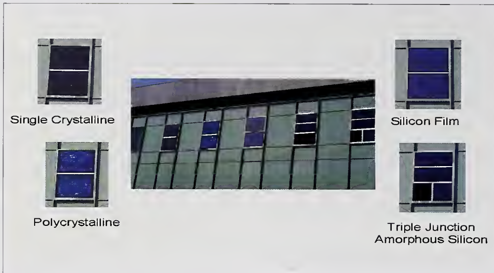
NIST's Building Integrated Photovoltaic Test Bed.
