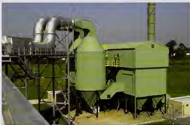
Newly installed pollution abatement system for the Large Fire Laboratory.
