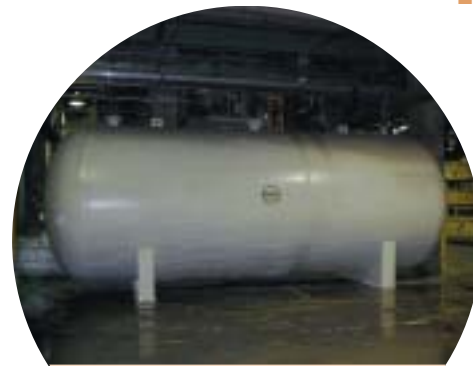
New 10,000-gallon compressed air storage tank
