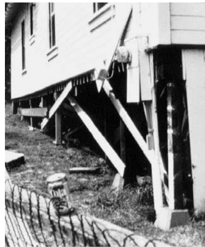
Figure 15 - The pier-and-post foundation under this home shifted during a recent earthquake.
