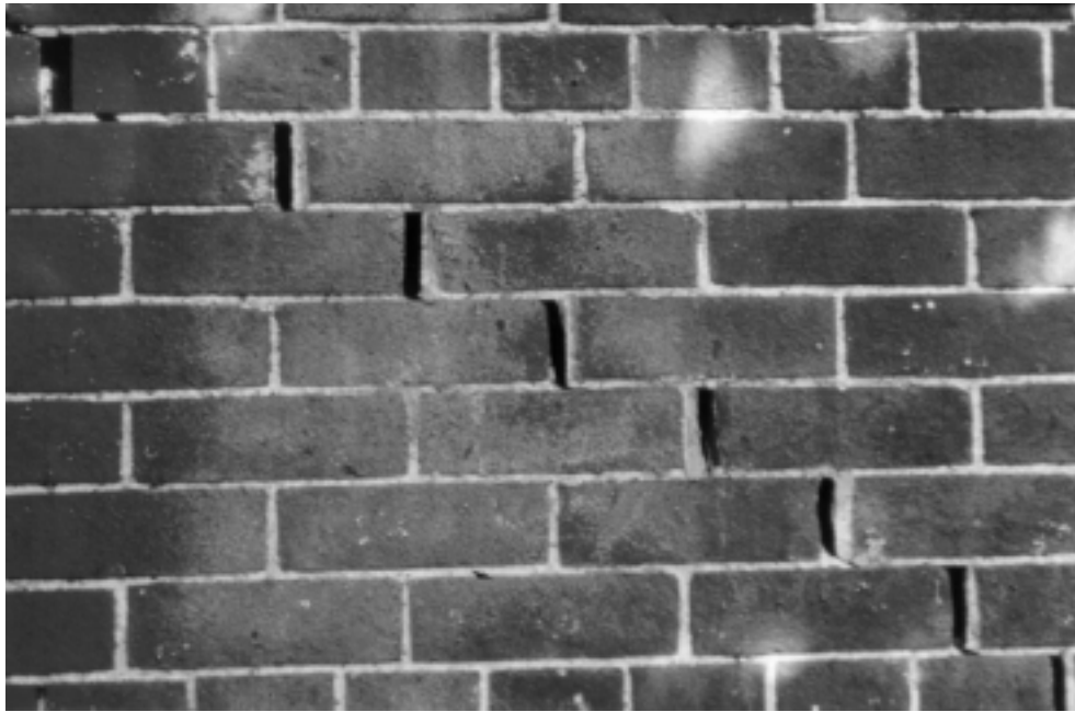
Figure 7-10 Photo of Bed Joint Sliding
