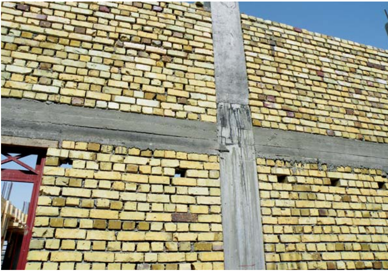
Basrah Modern Slaughterhouse under construction, showing upper-level concrete intermediate (cross) beams improperly supported by brick façade.
