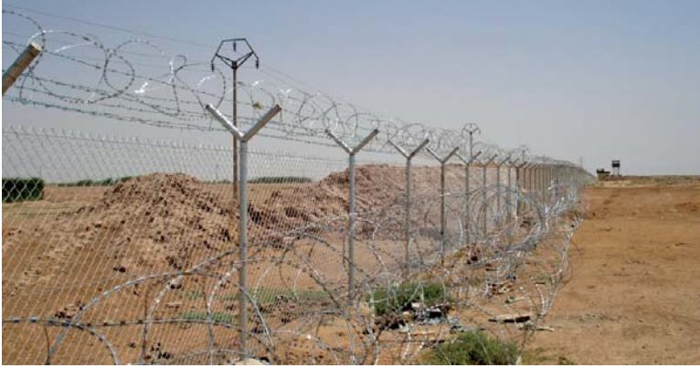
Chain-link fence and barbed wire along Phase 3 of the pipeline exclusion zone for the Kirkuk-to-Baiji pipeline.
