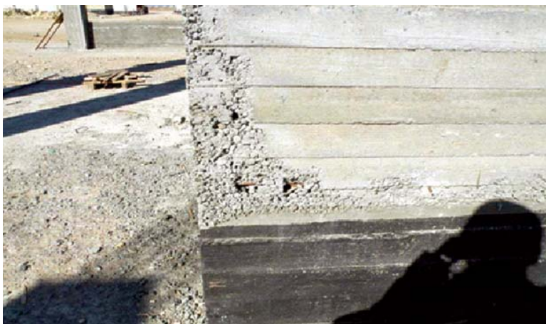
Unacceptable cement pour with honeycombing and exposed rebar at the Missan Surgical Hospital.
