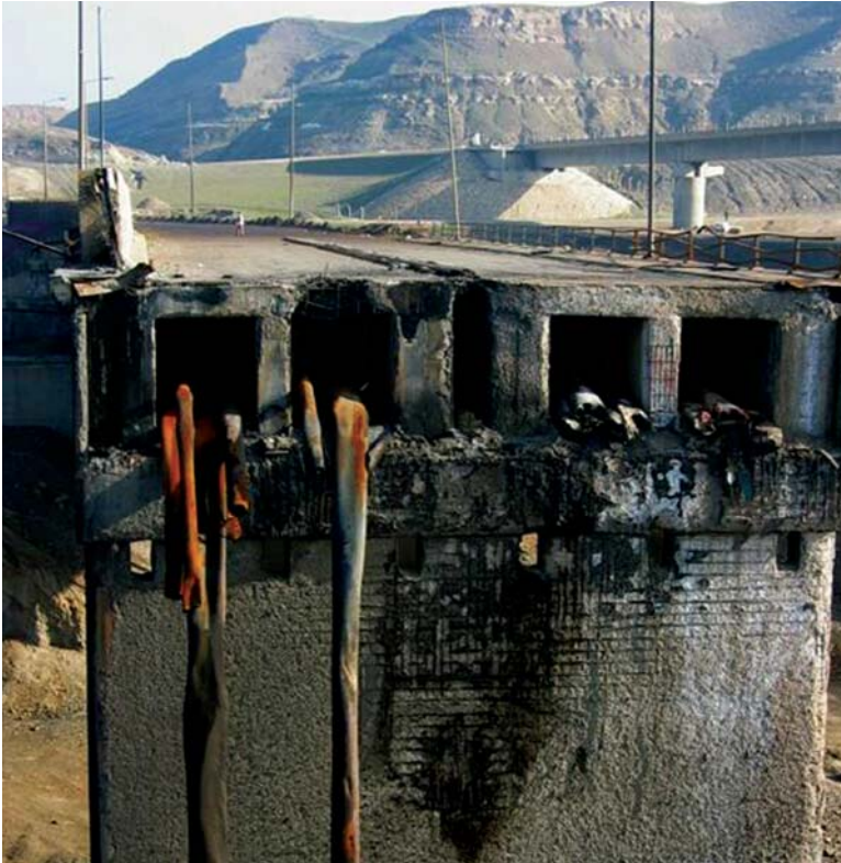
Cross section of al-Fatah bridge showing melted oil pipes. (USAID photo)
