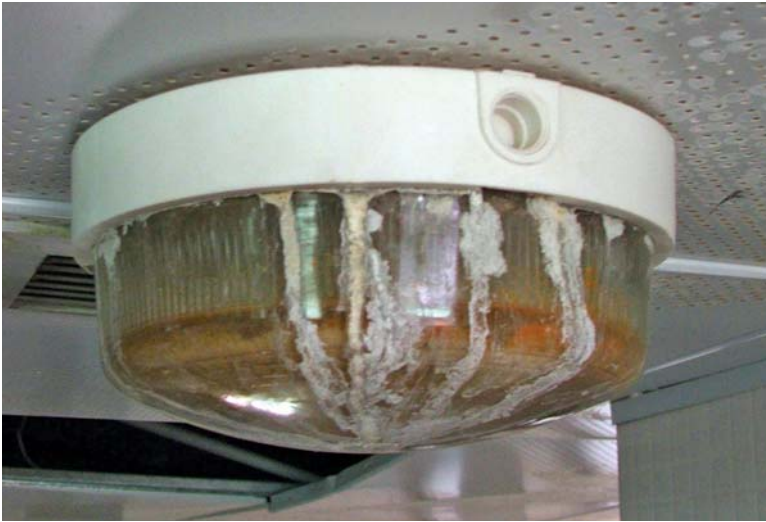
Urine-filled light fixture in cadet barracks bathroom at the Baghdad Police College.
