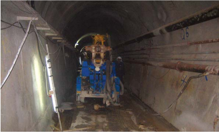
Grouting equipment in the tunnel under the Mosul Dam during SIGIR inspection.
