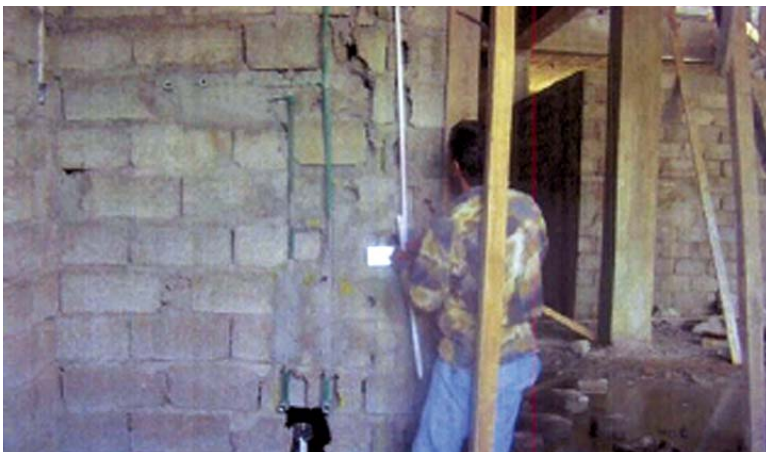
Example of poor block laying at primary healthcare center in Kirkuk. (USACE photo)
