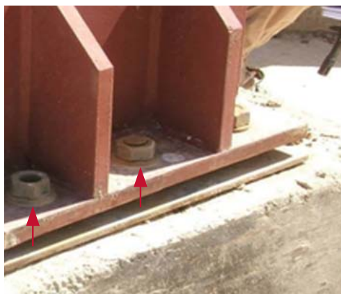
Example where one foundation bolt extends beyond the nut and another bolt does not.
