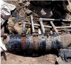
Illegal taps in the transmission and distribution lines, which reduce the water pressure and amount of water available to residents. (USAID photo)
