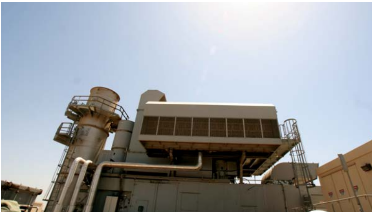
Frame 9E and LM-600 generator units at the Qudas Power Plant.
