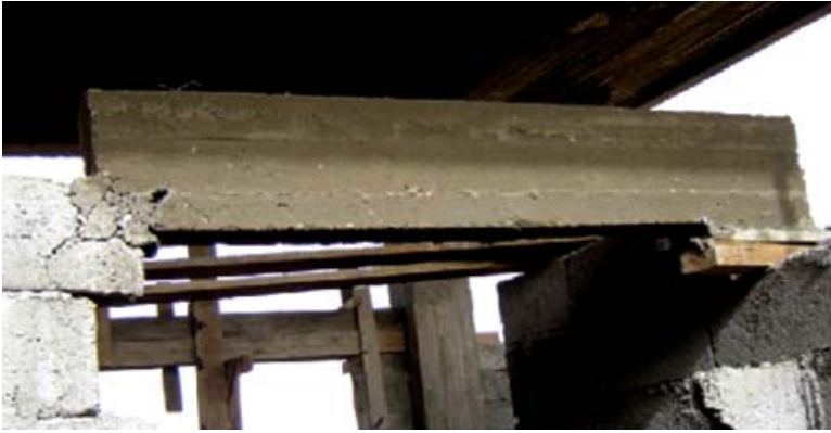
Improper support for a load-bearing lintel at a primary healthcare center during construction. (USACE photo)
