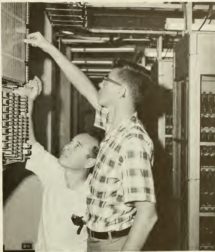
Peter W. Foster, left, leader Central Office repairman, and Frederick R. Walker, Central Office repairman, shown with new communications equipment that has been installed in the Administration Building. Foster, with 17 years Panama Canal service, is a graduate of the Canal's apprentice program, worked in Cristobal and came to the Pacific side office 2 years ago. Walker served his Canal apprenticeship in Cristobal and has been on the Pacific side about 2 years also.
