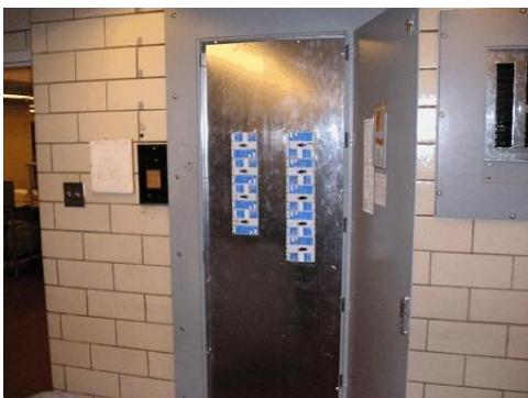
Figure 2b: Same electrical panel after abatement. This panel now has a “dead front.”
