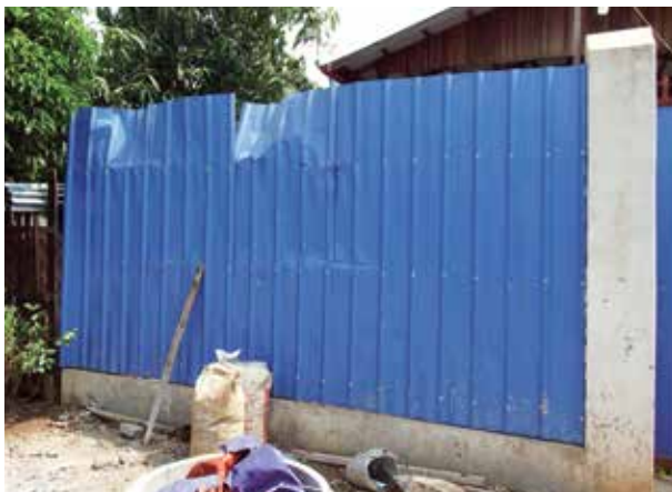
Damaged compound, Yesagyo. Photo: Rachel Fleming
