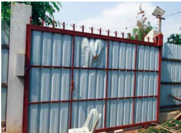
Damaged compound, Yesagyo. Photo: Rachel Fleming
